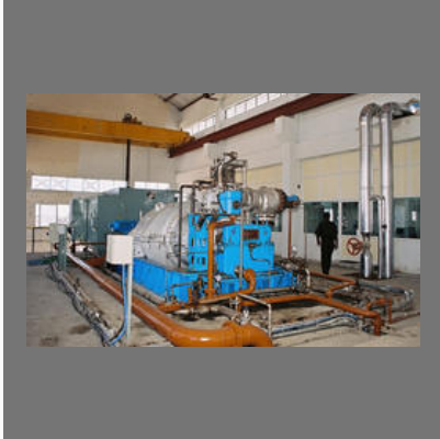
Extraction Condensing Turbines
