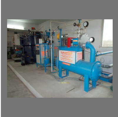
Steam Turbine Power Plant With Non Ibr Boiler
