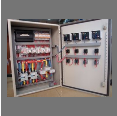
Electric Panel Boards
